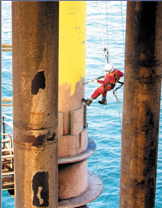
Rope Access Operative at work blast cleaning prior to spray painting a gas platform leg
